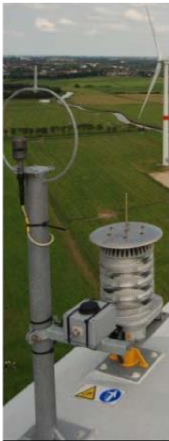
Fig. 4: Example of a lightning rod at the nacelle of the 3.XM-series
