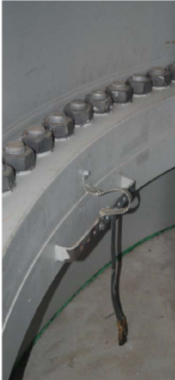
Fig. 7: Equipotential bonding busbar connection to the earthing system of the WEC
