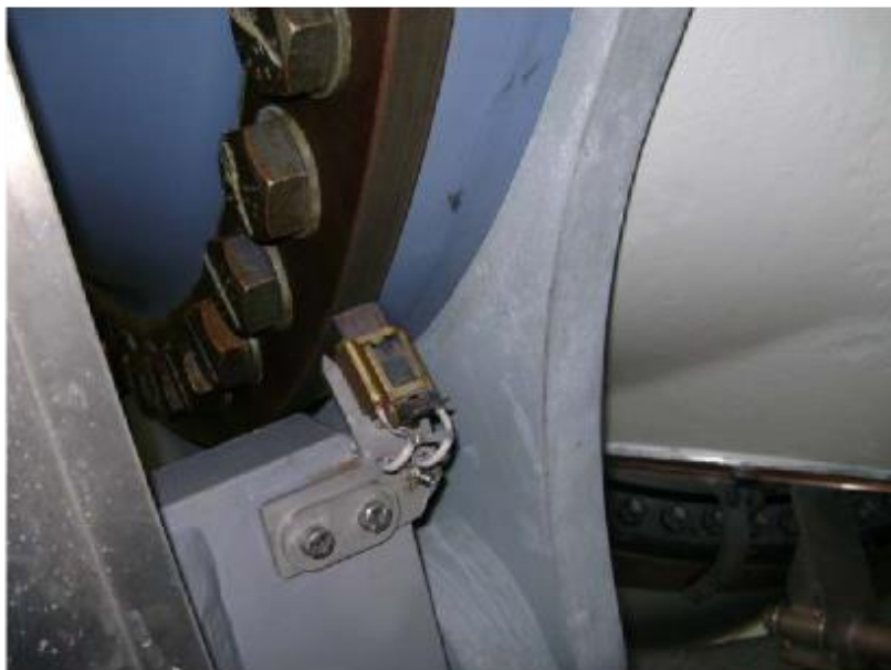
Fig. 3: Carbon brushes with parallel spark gaps at the rotor holding disk
